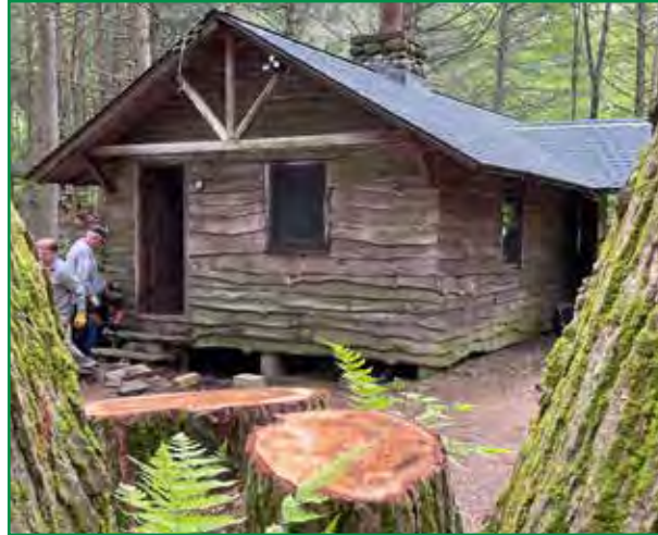
May 18, 2024 – Work party spruces up after tree work, new roof and outdoor security lights
